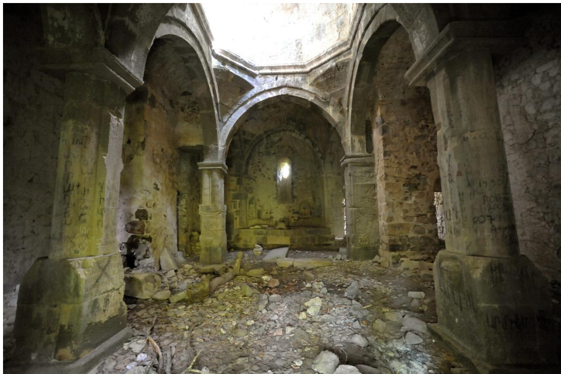
Figure 5.46. Khat'ravank' monastery (late 12th–13th century), Arts'akh. Narthex ( gawit' ), 1225. View of the interior in easterly direction. Photo: R. Kortoshyan
