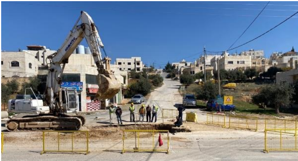
Building works on land purchased by a civil servants' cooperative in Amman, Jordan, 2021 © Kalaldehy
