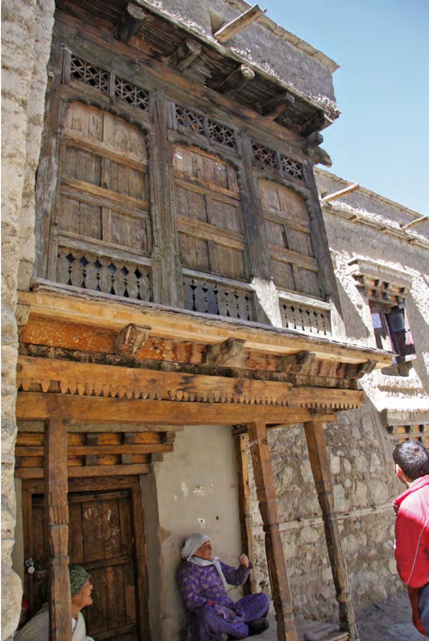
FIGURE 5 The Sofi House, dating from the early nineteenth century, shows the beautifully carved wooden doors and balconies typical of a Kashmir-style house. The rafters, beams, and pillars are made of poplar.
