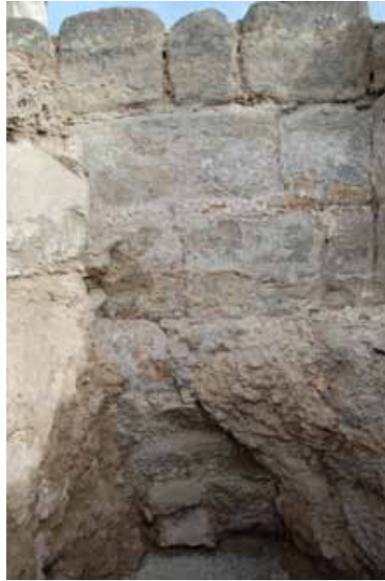
Fig.21: Detail of the foundation under wall M4 in B2 after having removed the mortar (JB 2014).
