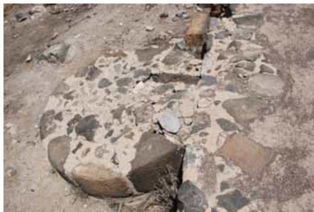
Fig.49: Detail of the restored buttress 12-4e with the continued facing of wall M3 (AS 2014).
