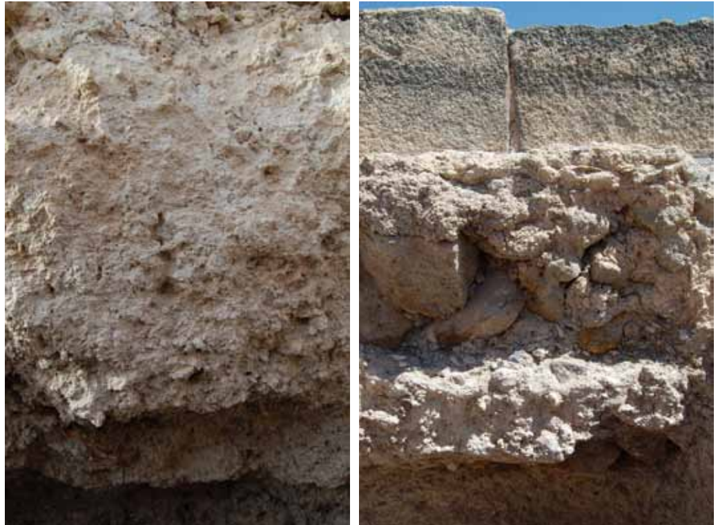
Fig.46: Detail of the mortar in sounding G2 Fig.47: Detail of the different layers of the foundation in sounding G2 (JB 2014).
