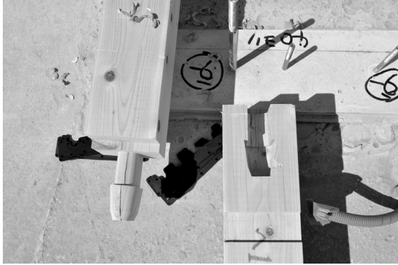
Fig. 18: Mikan, EFEO Centre Kyoto, joints between two beams, September 2013. Photograph ©Benoît Jacquet.
