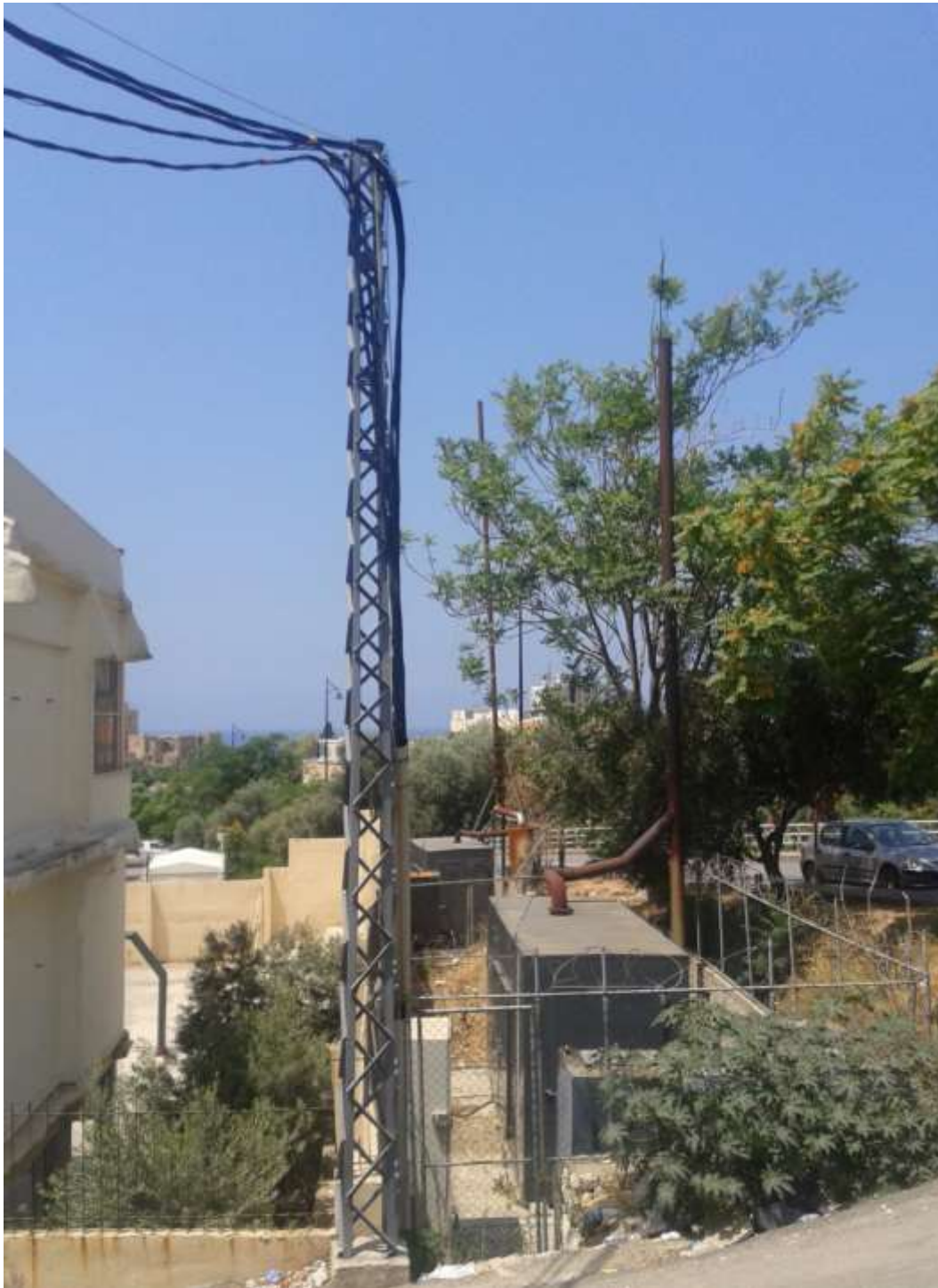
Figure 17.3 A fenced generating unit belonging to EDJ, and a pole in the grid managed by the same company.
