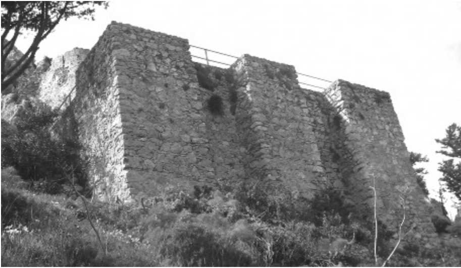
Fig. 7. ABOVE: - Cistern in Kantara; Cl. N. Morel, 2008. This enormous cistern, supported by three buttresses, is built outside the enceinte, below the castle, to optimise water reception. Built perhaps for providing for a considerable number of soldiers when the castle housed a garrison in the late 14th century, the tank reflects the importance of water in the region.
