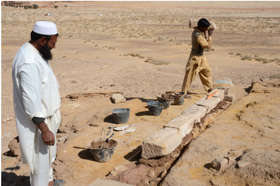
Fig. 4. Restoration of the northern wall of the enclosure surrounding the top of IGN 132.
