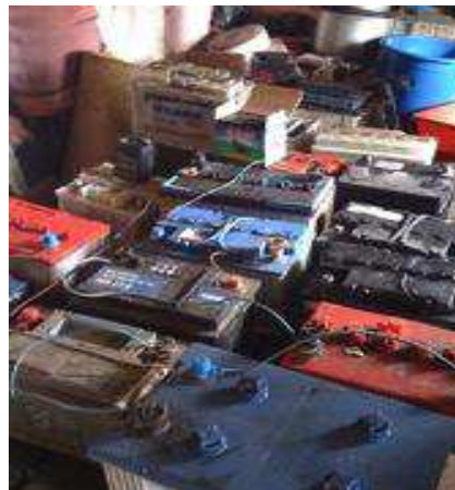
Batteries continuously connected for recharging
