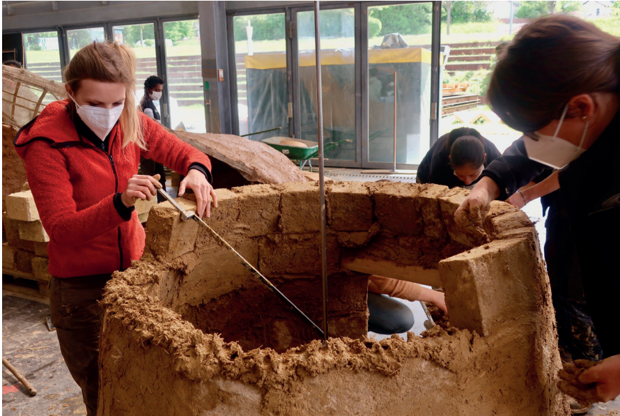
Figure 5. Bricklaying the mud-brick courses with the help of the mechanical arm. © María Lidón de Miguel.
