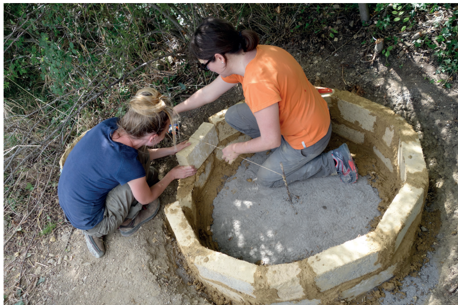
Figure 7. The second silo prototype. The bricklaying of the first mud-brick courses. © Aurélie Feuillas.
