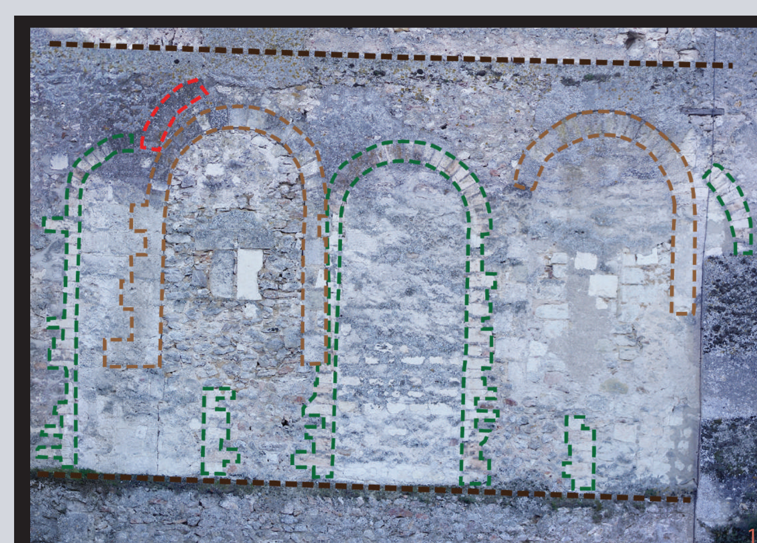
12 - Projections and plugged windows on the east face of the St Paul tower.
