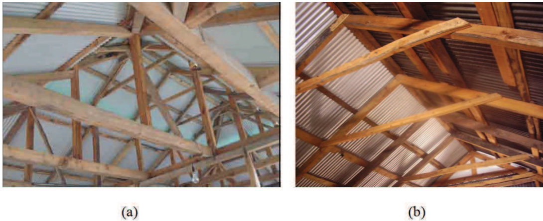
Figure 6.44 — Frame of tower roof. (a) Source : UNHABITAT, Unpublished Draft, 2012 ; (b) Source : S. Abidi
