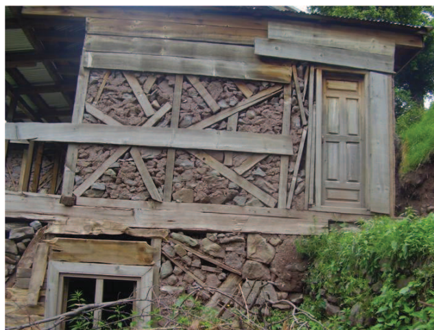
Figure 7.35 — Example of large distance between studs, under/over sized bracings and lack of connections. Although upper floor was treated with remedial measures, lower part has connection issues. Source : S. Abidi
