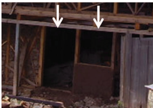
Figure 8.7 — Issue of openings. Source : S. Abidi
