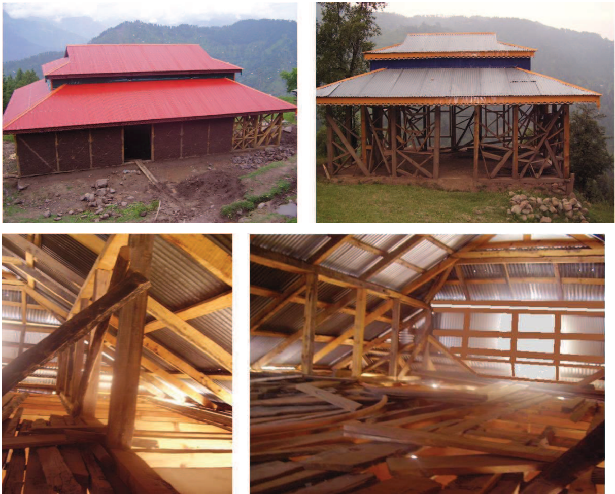
Figure 6.60 — Exterior and interior views of different under-construction houses in Muzaffarabad. Source : S. Abidi
