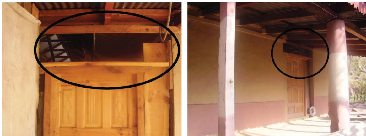
Figure 7.3 — Open spaces on top of the doors. Source : S. Abidi.
