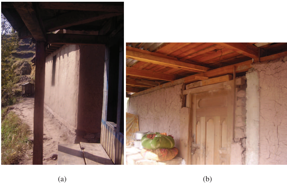
Figure 5.28 — Mud plaster is frequently applied on the walls. This not only avoids rain water seepage but also provides thermal insulation to some extent. Source : S. Abidi.
