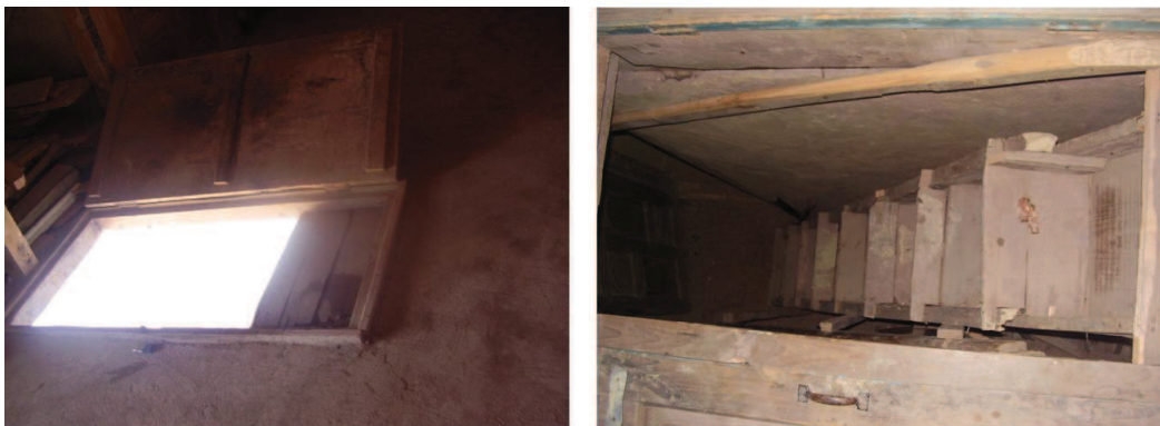
Figure 6.77 — The punctures in the ceiling to access tower roof. Source : S. Abidi
