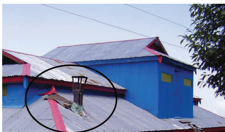
Figure 7.18 — As leakage from around the chimney was to be avoided, the owner has just put a small piece of CGI sheet and then put stone. Plastic is also surrounding the chimney. The owner was still facing water seepage. Source : S. Abidi
