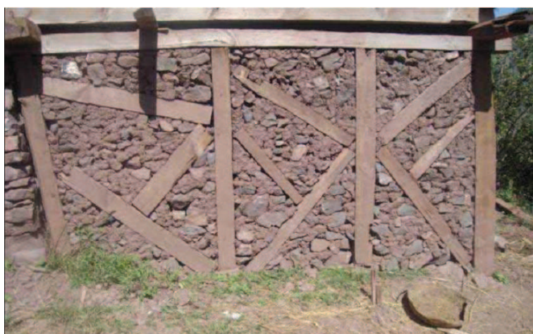
Figure 7.33 — Non compliant construction due to size of bracings, larger distance between studs and poor connections. Source : [Schacher, 2006]
