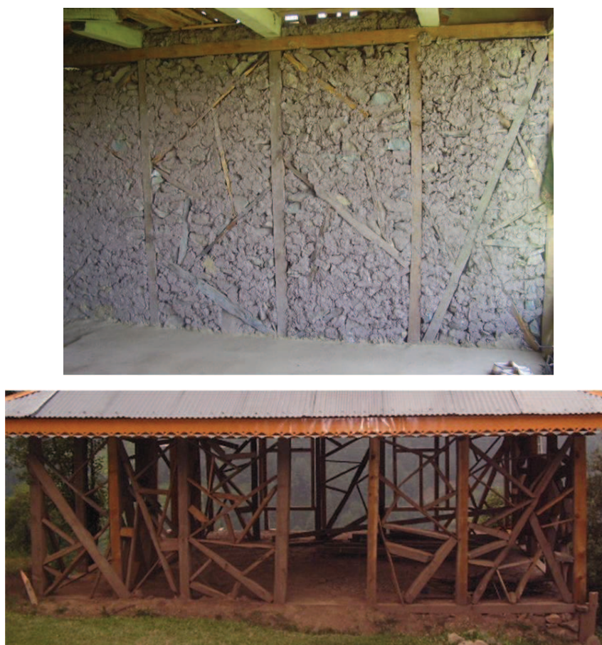
Figure 8.23 — Retaining wall and bracing members issues. Source : S. Abidi
