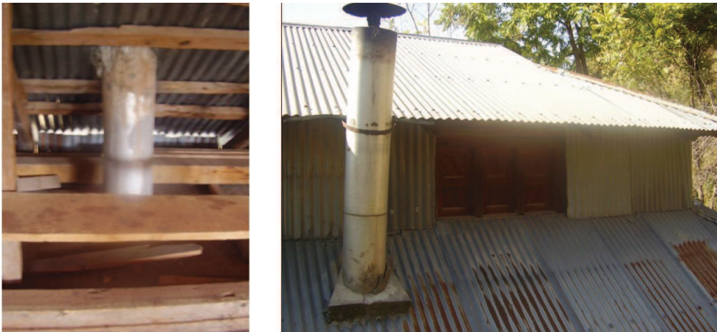
Figure 6.67 — Left : venting pipe passing through the eaves. right : the same pipe projecting out. Source : S. Abidi
