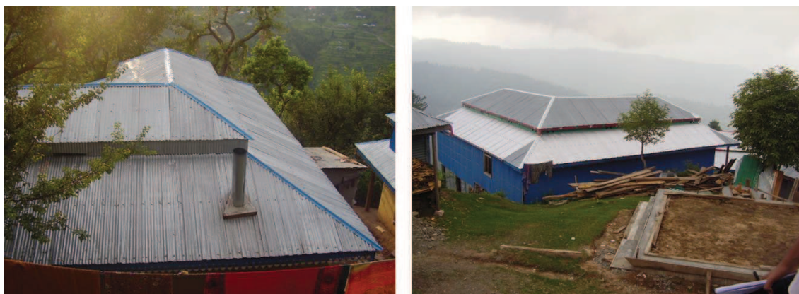
Figure 6.32 — Negligible break hip and valley roof. Source : S. Abidi
