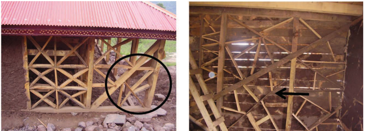
Figure 8.16 — Plinth and bracing member sizing problem. Source : S. Abidi
