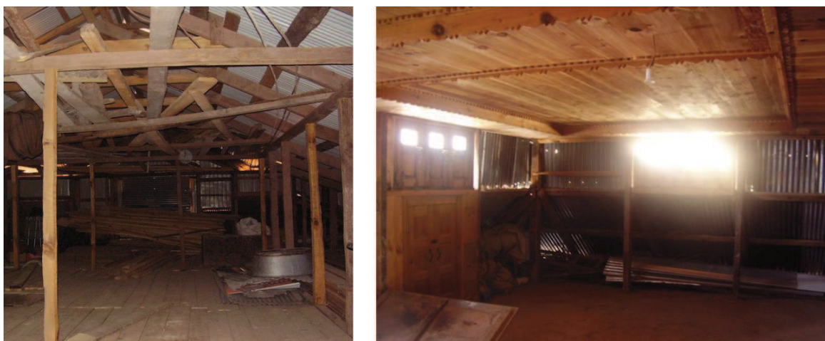
Figure 6.50 — Left : Pitched roof can be Seen from inside ; Right : Ceiling is added in tower roof. Source : S. Abidi
