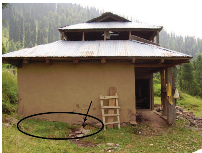
Figure 7.25 — Direct contact of walls with the ground. a hole is observed in the wall due to water seepage. Source : S. Abidi
