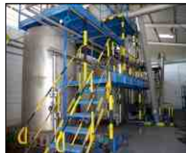
Photo 143 – Atelier de distillation
