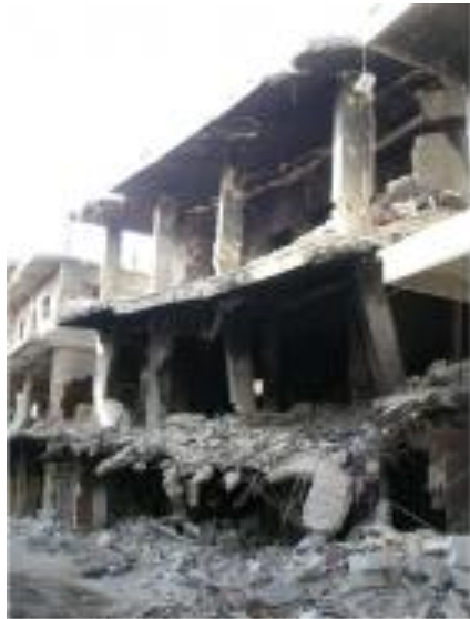
A damaged building, new camp, Nahr el-Bared, November 2007.
