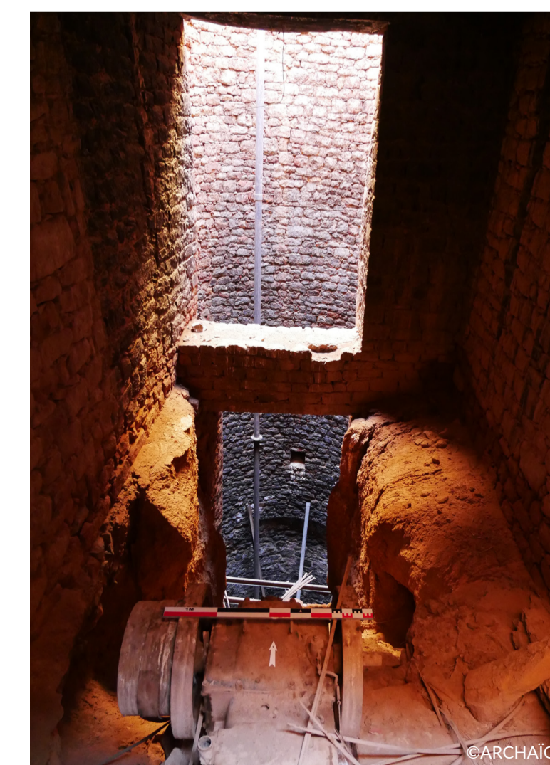
The well OS_08568 from the lower machine room, looking north. We can see the reused rails in the pit to support the pumps but also as lintel for the openings.
