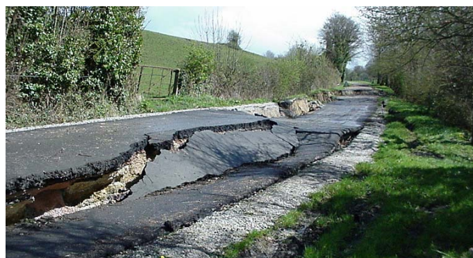
Figure 1. Example of a damage induced by a landslide triggering in the Pays d'Auge plateau (Source: TP-Geo)
